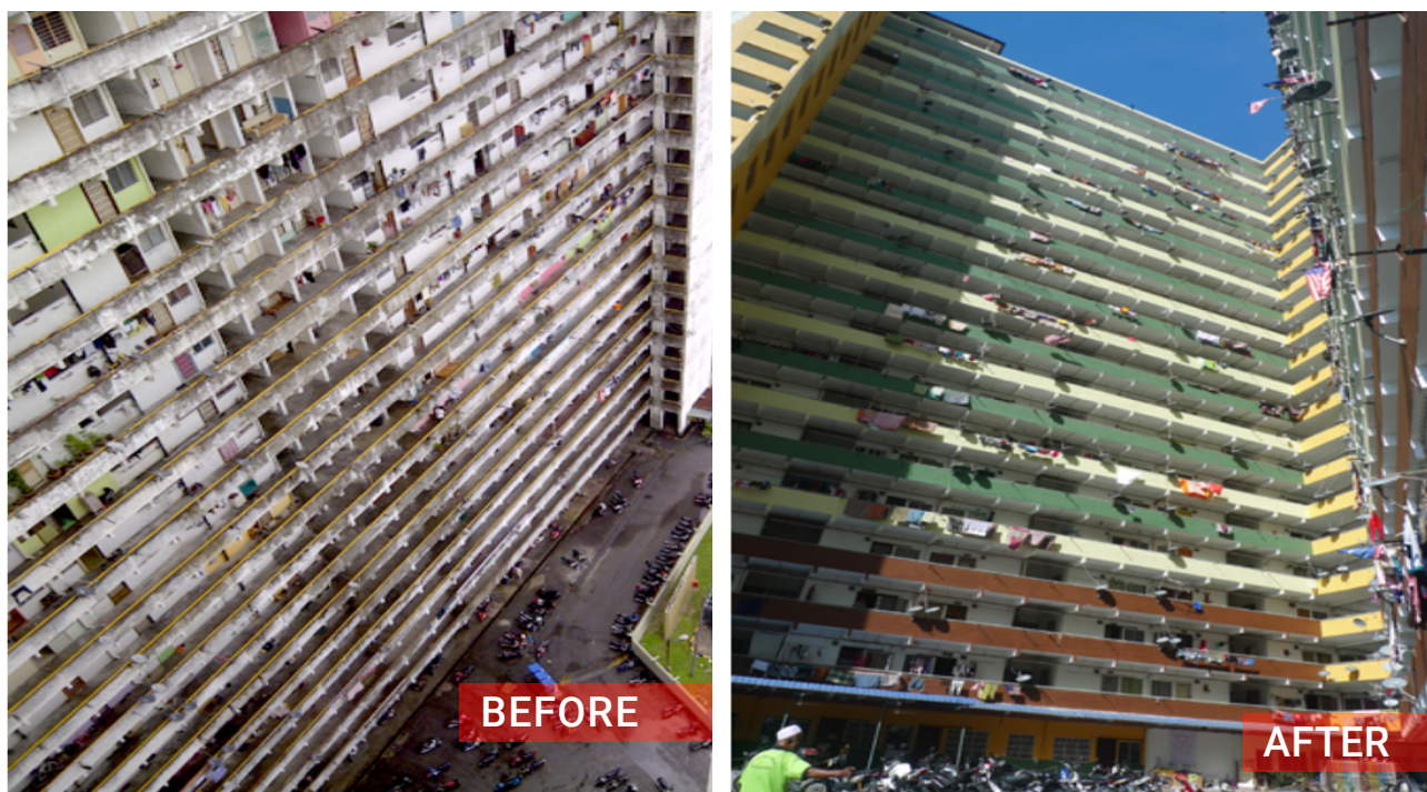
Picture 11. Jalan Sungai Flats, Penang, before and after PB Credit: Shariza Kamarudin, WPDC, 2014
